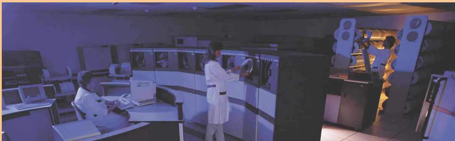
Data centre: Security application
